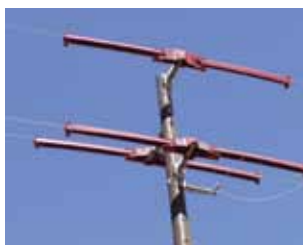
2 Pieces: MVLC-38 on busbar with BCIC
