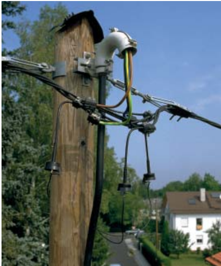
Transition: insulated overhead lines to cables
