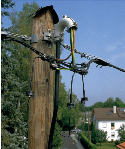
Transition: insulated overhead lines to cables
