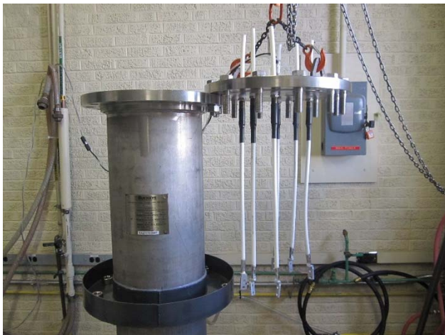
Figure 21 – Cable Assemblies Secured to Pressure Vessel Lid
