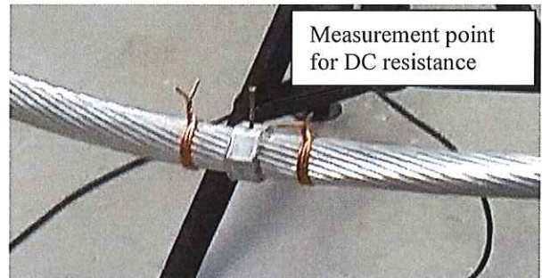
795 kcmil AAC Control Conductor
