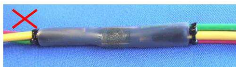
2. Overheat of tubing
