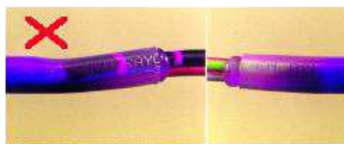
2. Overheat of tubing
