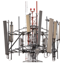
Remote Radio Units (RRU)
