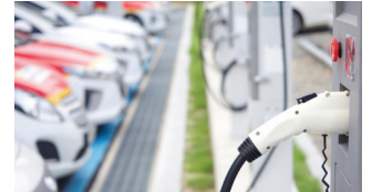
Electric Car Charging Stations
