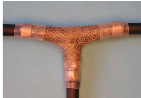
NOT ACCEPTABLE Insufficient solder flow
