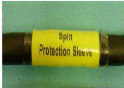
NOT ACCEPTABLE Split Protection Sleeve
