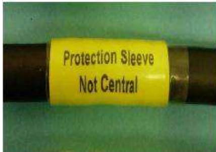
NOT ACCEPTABLE Protection Sleeve Not Central
