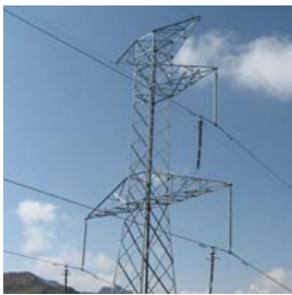
Transmission line arresters
