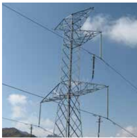
Transmission line arresters
