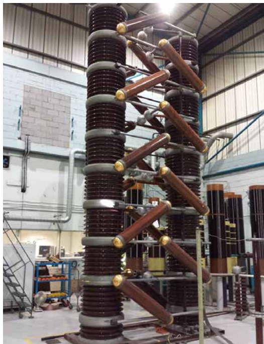
MARX impulse generator 1.65 MV
