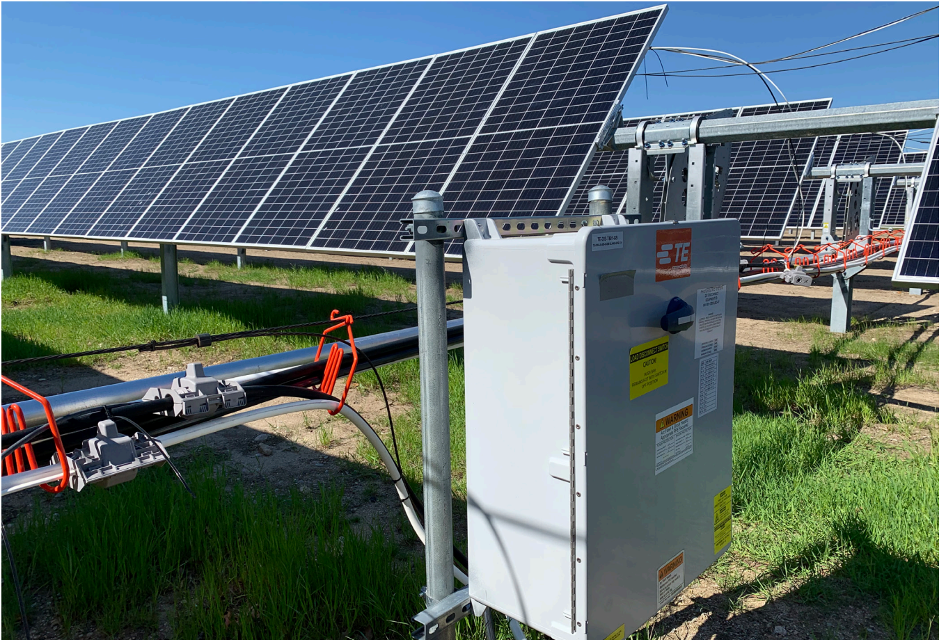
Solar IPCs and Disconnect Box
